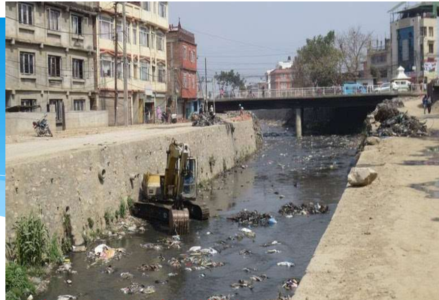
Drainage and wastages in Dhobi khola Source: Raj Maharjan
