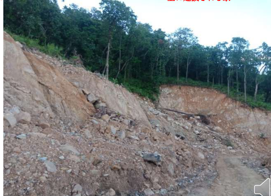
Non-engineered slope for road construction Source:Spotlight Nepal
