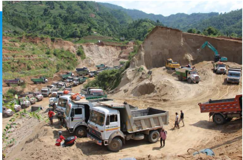
Sand mining near settlement Source : CIJ Nepal 居住区域付近における土砂の採掘
