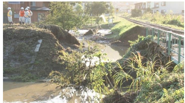
Fig. 8 Site of Sara-gawa River Collapse (Oct. 14 th )
