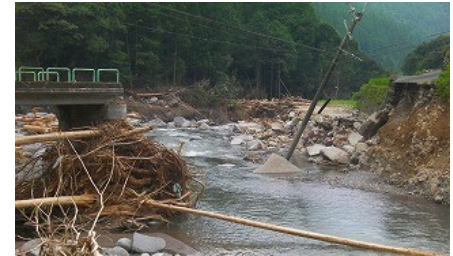
Flow out of bridge's girder by heavy rain
